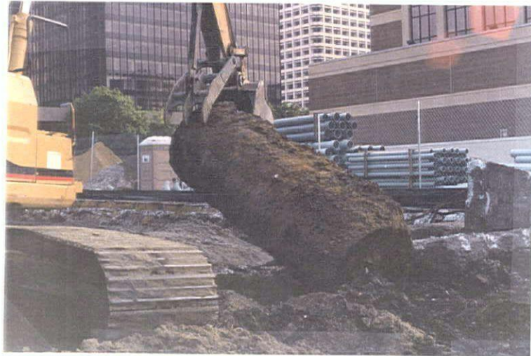
Top View of UST 3
