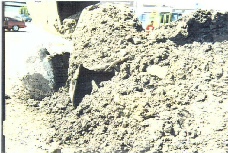
Top View of UST 1.
